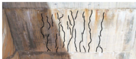
Flexural Cracking Example
