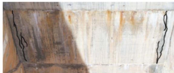
Shear/Tension Cracking Example
